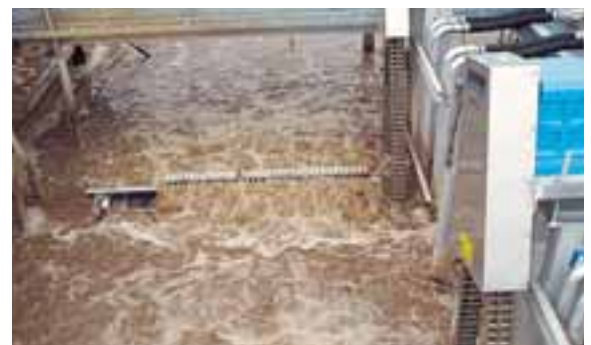
Industrial WWTP Raisio Chemicals with 2 VRM® 20/198 units, extendable to 2 VRM®20/252 units, with 1512 m 2 total membrane surface
