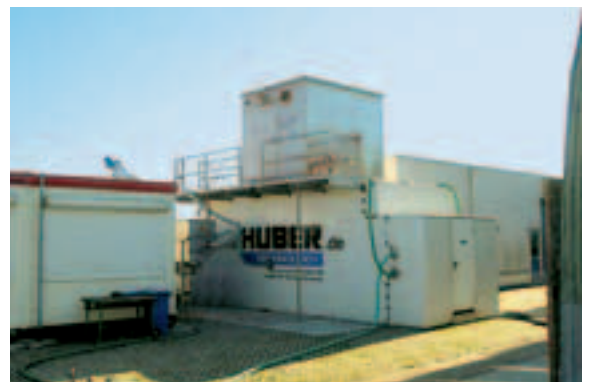
Membrane Bioreactor pilot plant (Netherlands)
