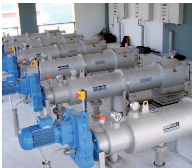
Sludge screening on WWTP Athens, Greece
