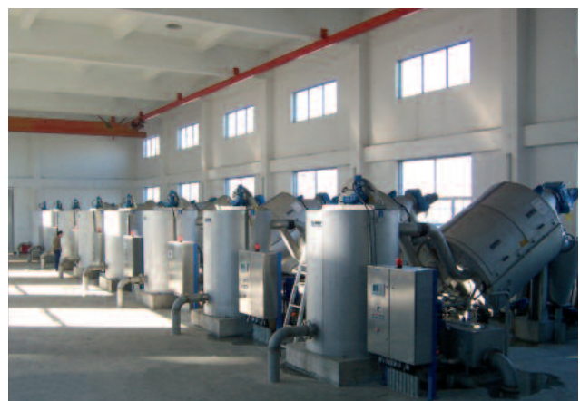
Eight screw thickeners handling 600 m 3 /h
